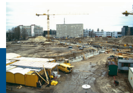
Excavators and cranes roll in to dig the ground for the storage ring.
