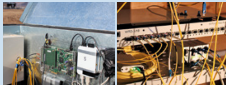
Figure 3: Nanosecond-Timing Units (White Rabbit) installed in HiSCORE stations (upper) and in the counting room (lower). Image by DESY
